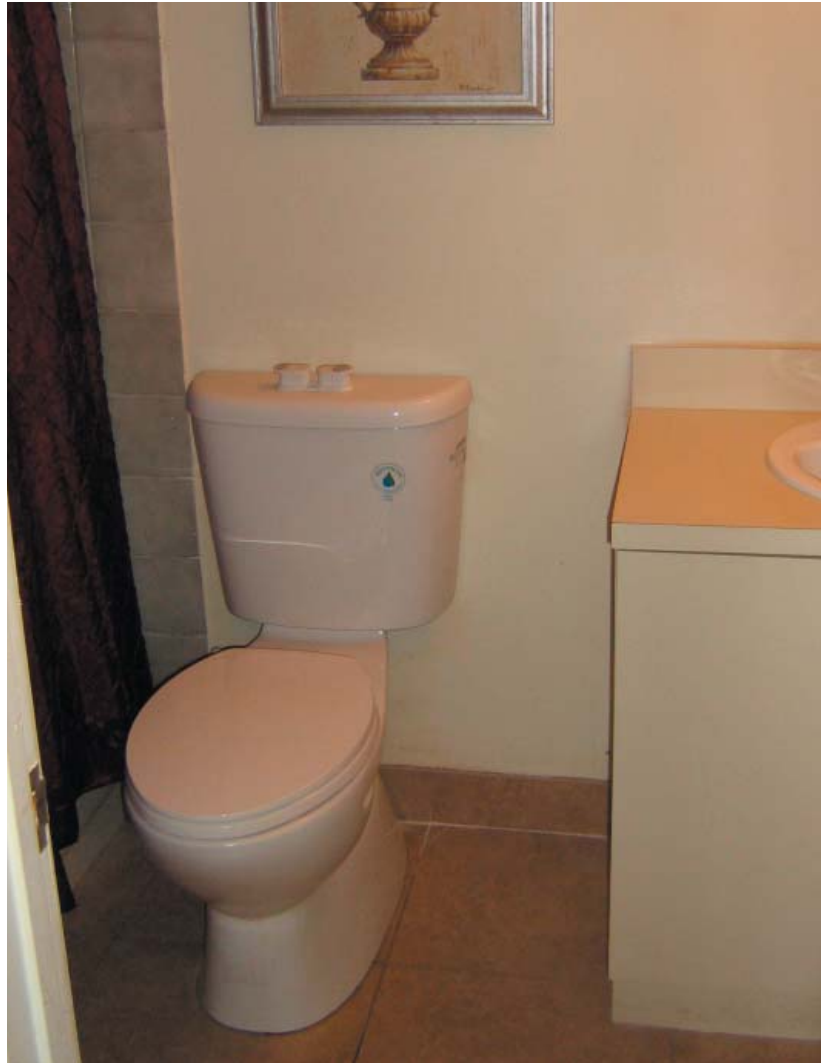
Image 1: Sydney installation at College Gardens Apartments
